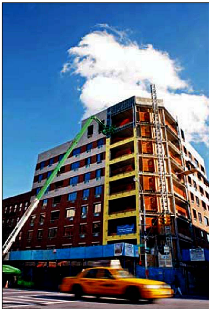
A new apartment building is under construction at West 114th Street and Frederick Douglass Boulevard in Harlem. (JIM COLESON/IMNY)
